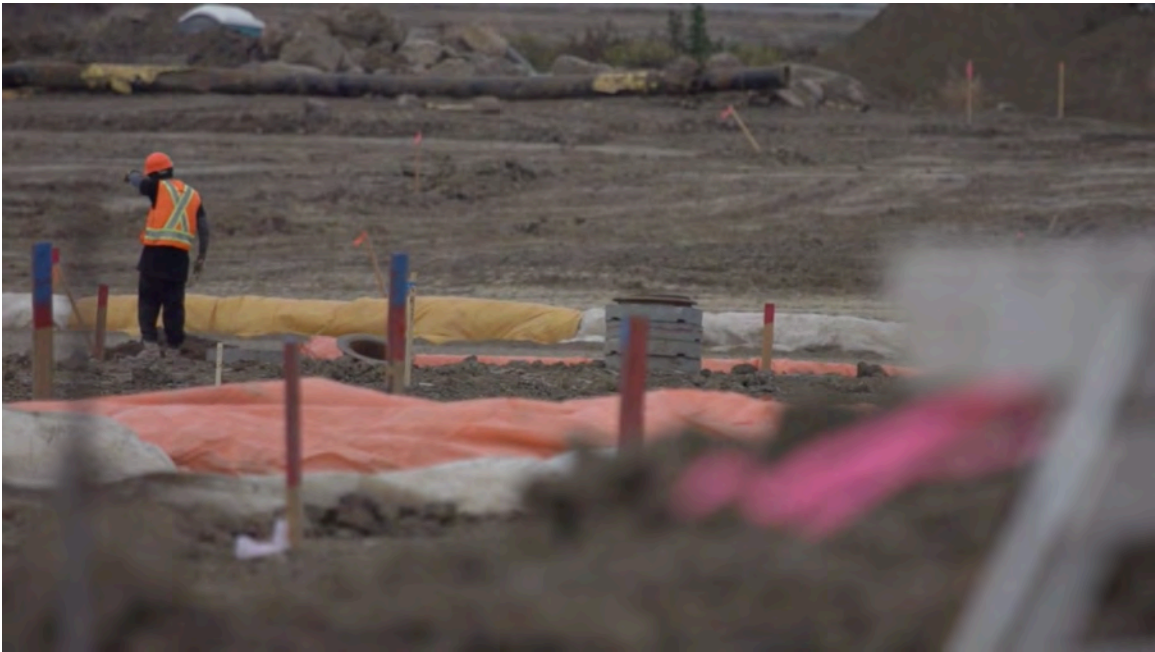
Fig. 36. Andrew Denton. [Film Still: Crude ] Worker on Construction Site, Edmonton, Alberta, Canada (2013).
