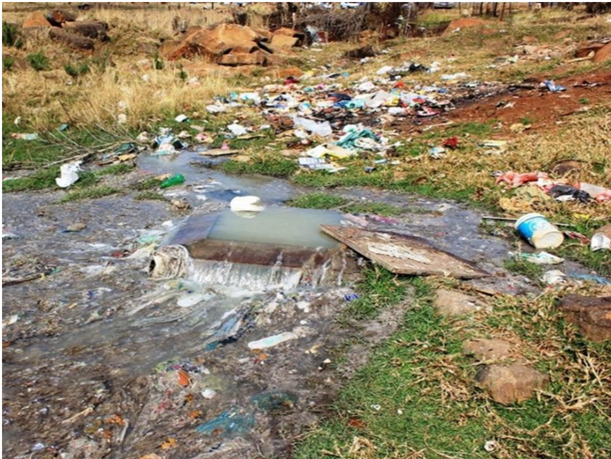
Figure 4.2: Spilling manhole and illegal dumpsite in Mpophomeni ( photograph from Kolbe 2014 cited in Ward, 2016 ).
