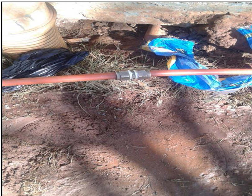
Figure 4.3c: The fixed water leak ( source author )
