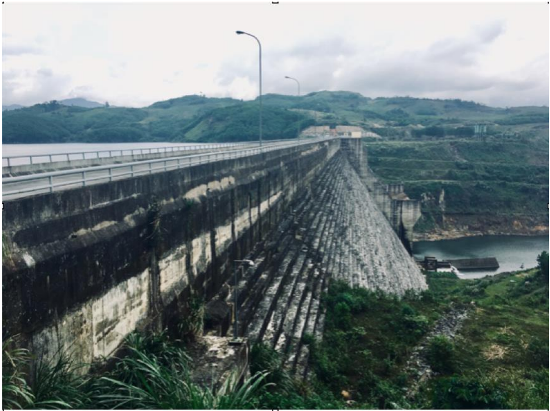
Figure 4.1: A section on the main dam of Song Tranh 2 Hydropower Plant (The photo was taken on 24th February 2017 in Tra Doc Commune, Bac Tra My District, Quang Nam Province, Vietnam)
